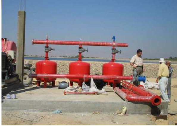
Figure 3 Filtration system (sand and disc)
